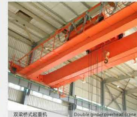
双梁桥式起重机 Double girder overhead crane
